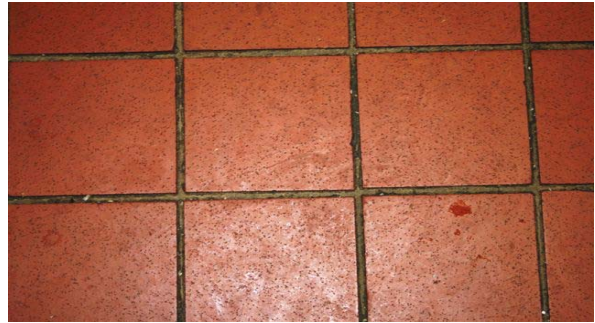
Grout in kitchen tiles starting to lighten with Chrisal use
